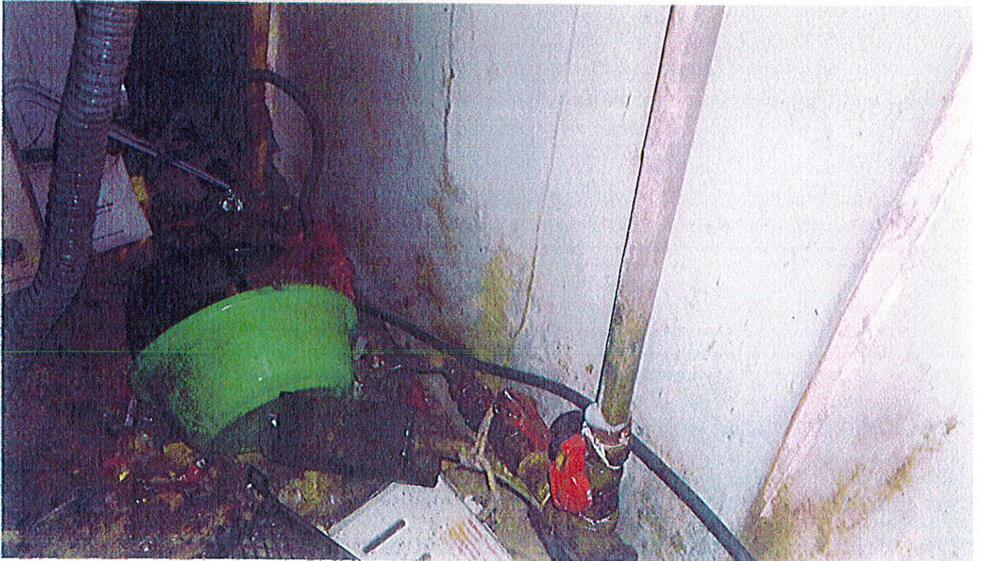
Gas leak #3 side in kitchen
