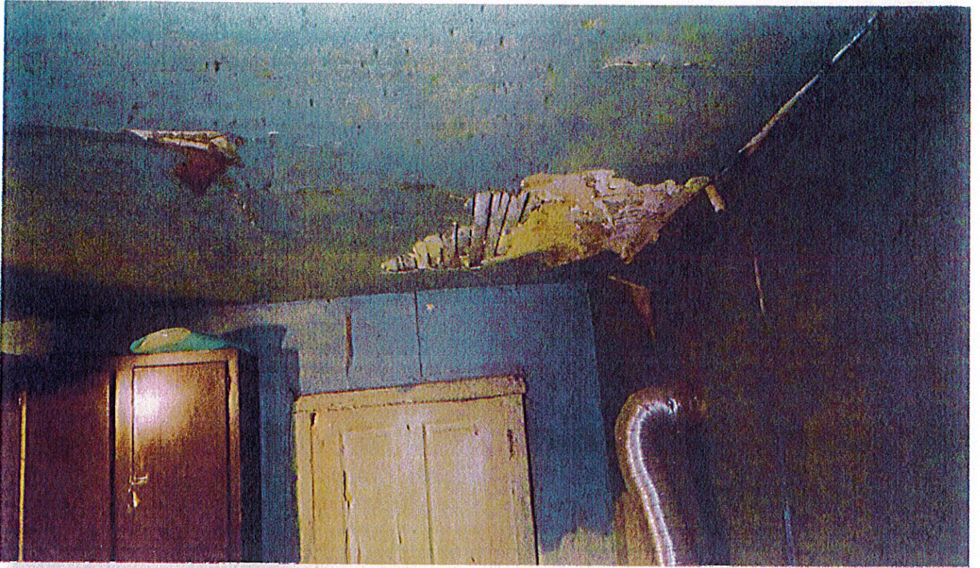
# 3 side kitchen and improper venting of gas dryer in kitchen
