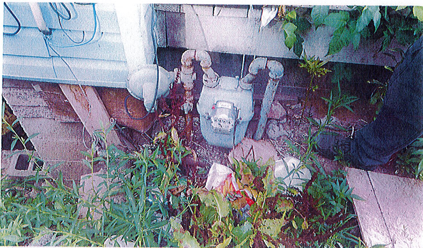
Gas leak at meter and service line #3 side
