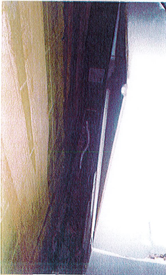
#5 gas leak behind kitchen stove
